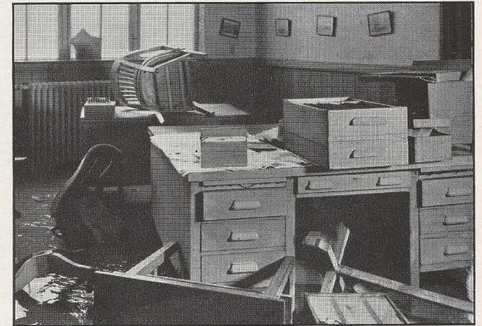
Ford Motor Co.—showing the interior of the office after the flood waters had subsided
